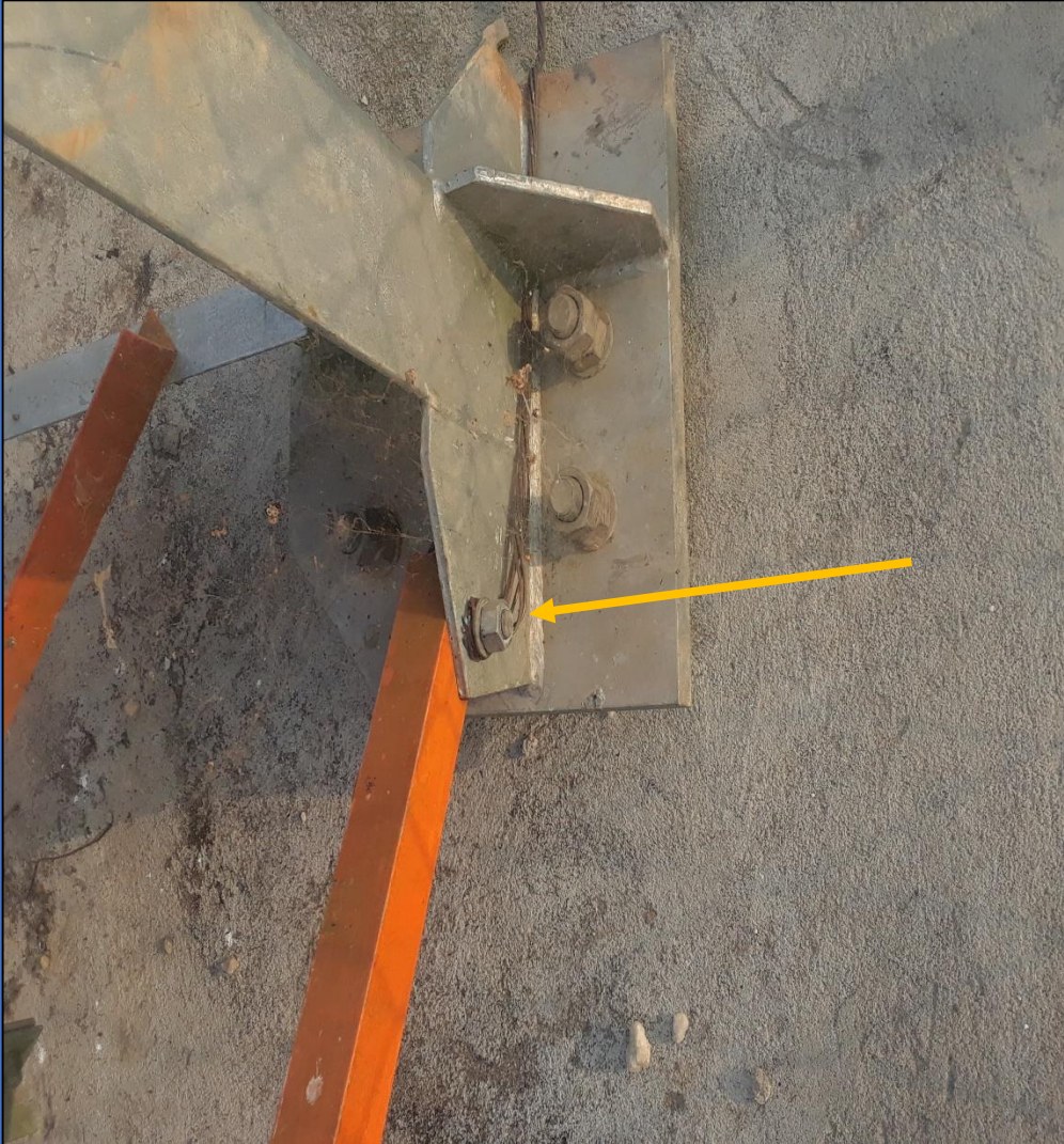
Grounding on tower leg has no cable lug.
