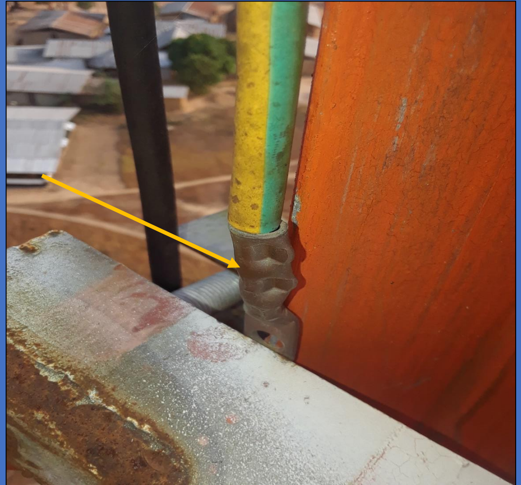
The Grounding cable is not terminated to a bus-bar. The tower has no bus-bar.
