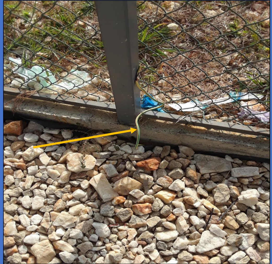
Grounding cable for the fence is 16mm 2 , not the standard for outdoor.
