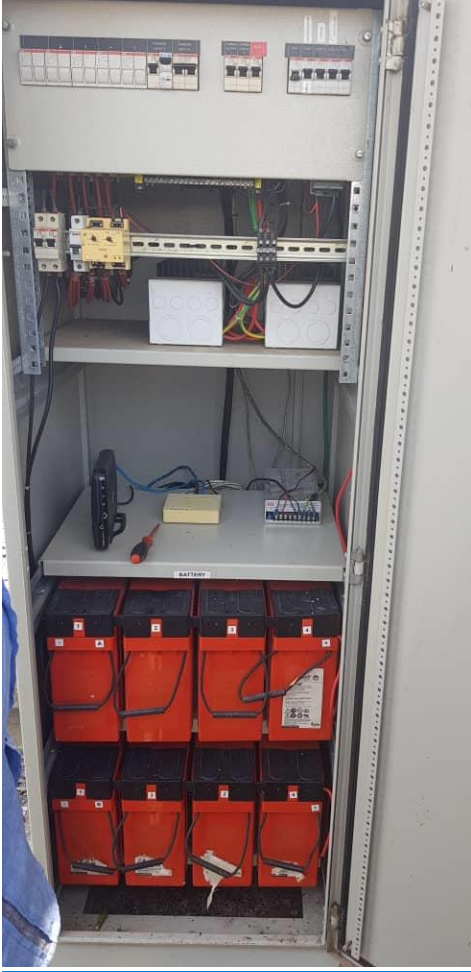
Figure 9 Battery component at Base station in Adidome
