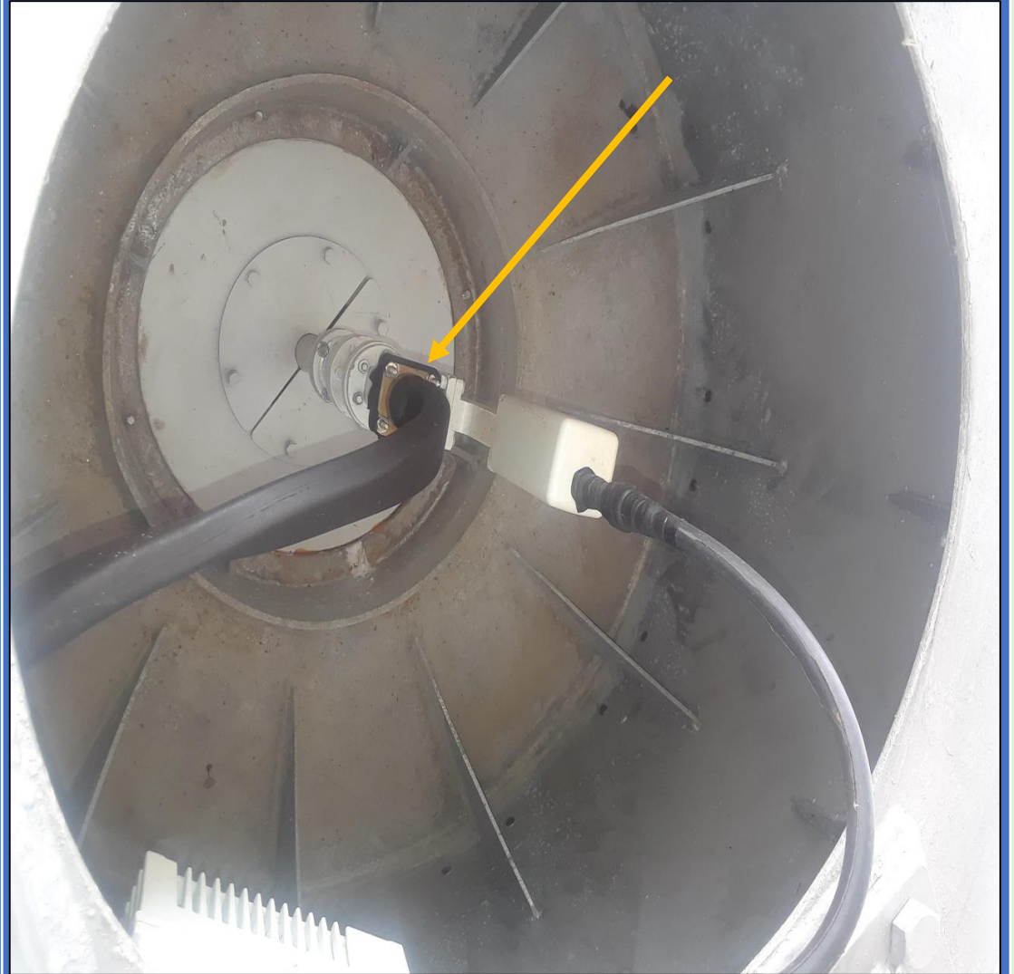
Waveguide is not protected with putty and tape.
