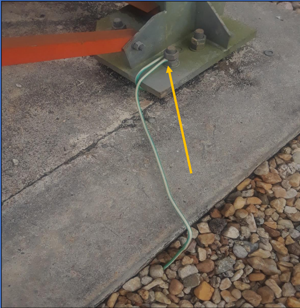
Tower leg wrongly grounded and no cable shoes.
