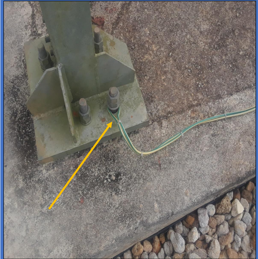
Tower leg not grounded.
